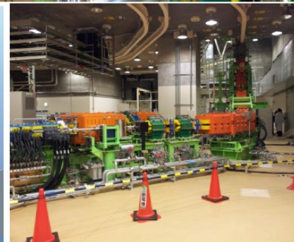
Extraction and beam transport
